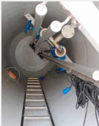
Pumpestation for dykkede pumper
